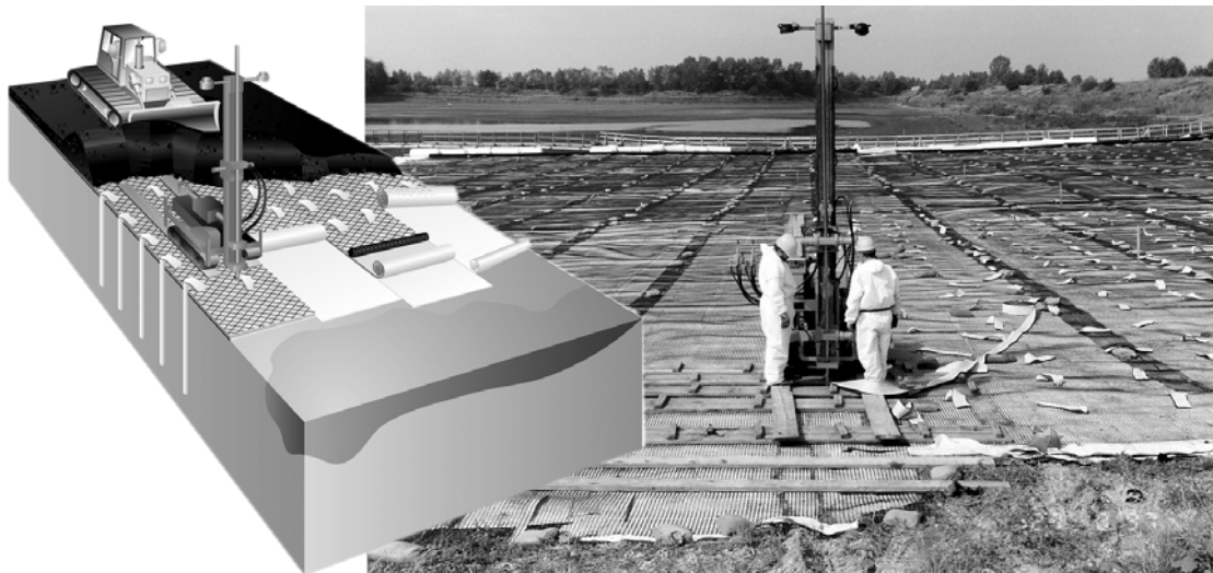
Fig. 7: Technology used to stabilise tailings impoundments, installation of vertical drains on the Trünzig tailings pond, subsite of Seelingstädt
