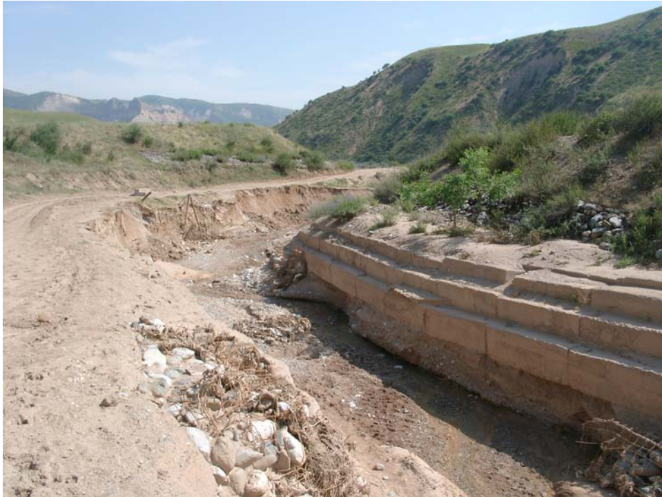
FIGURE 1. Fluvial erosion of the dam toe of tailings pond no. 2 and 13 in the valley of Aylampa Sai, a tributary of the Mailuu Suu river.
